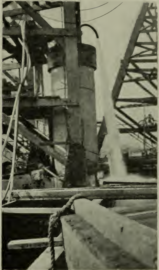
NEW HARBOUR WORKS AT VANCOUVER: CYLINDER IN PROCESS OF SINKING. (See p. 660.)
